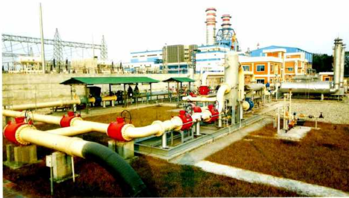
RMS of 360 MW CCPP at Bheramara
