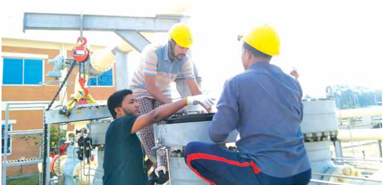
Bhola 225 MW RMS Maintenance
