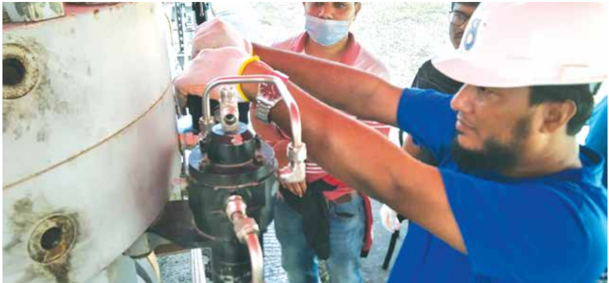
Bheramara CCPP RMS Maintenance
