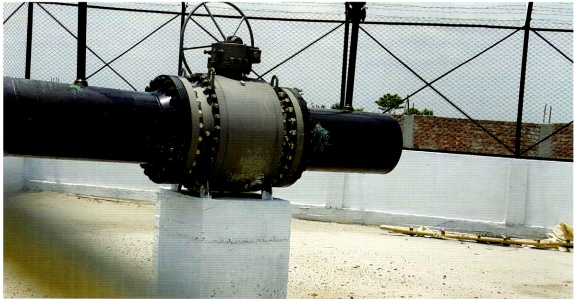
Valve Station at the Bank of Rupsha River
